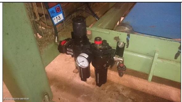
Ny installert FRL enhet.
